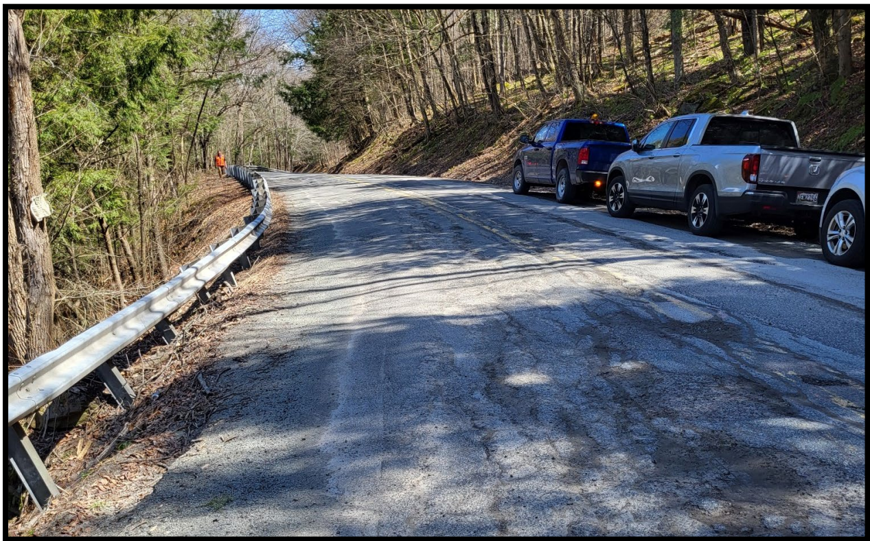
Figure 2: Pavement distress and tilted guide rail photo
