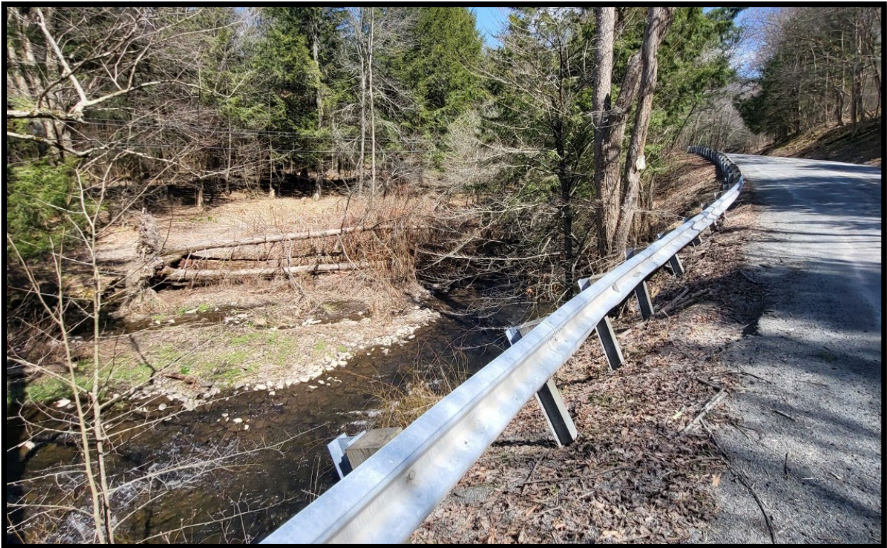
Figure 4: Gravel bar and stream at embankment toe photo
